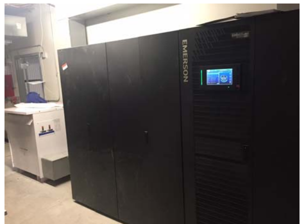
200kVA Power Center™ distributes EMERSON UPS output power to Gaming Machines
