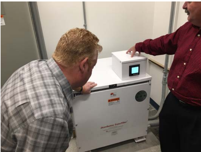
Rick Lopez, PQI's Director of Sales demonstrates the Type TPM Transformer Performance Meter to Clark County School District's Facilities Department
