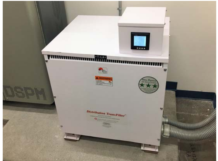
Ultra-Efficient e-Rated® Distribution TransFilters™ Installed in Clark County School District facility
