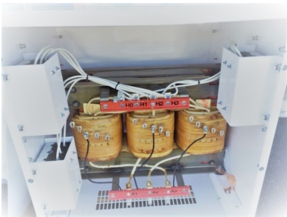
Type PC Power Center™ with three Side Mounted Feeder Circuit Breakers
