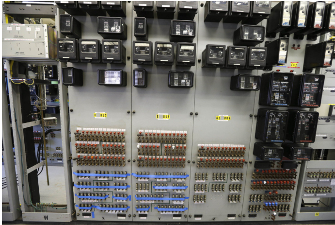
Typical Medium Voltage Feeder Circuit Panels with GE Type IAC 50/51 & 50/51N Protective Relays
