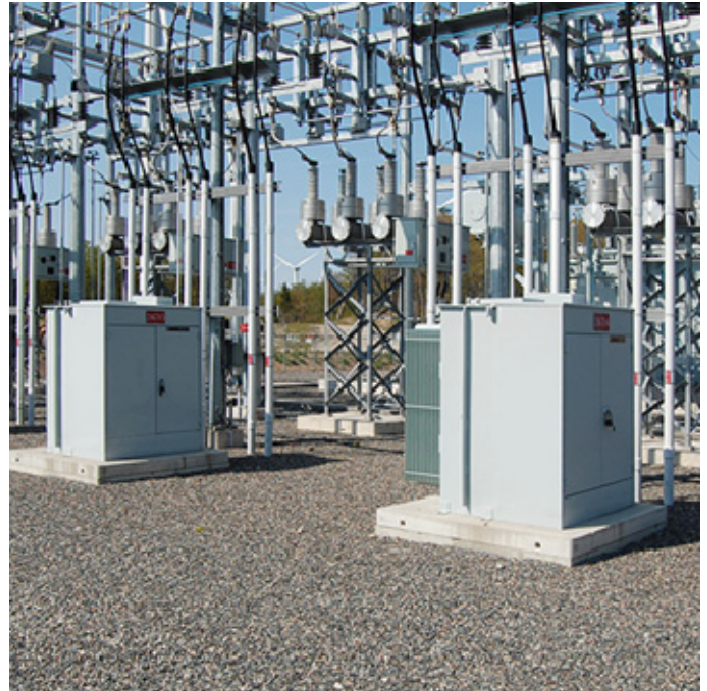
Transformer Station's Medium Voltage Yard
