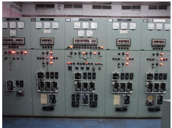
Typical Medium Voltage Feeder Circuit Panels with Westinghouse Type CO 50/51 & 50/51N Protective Relays
